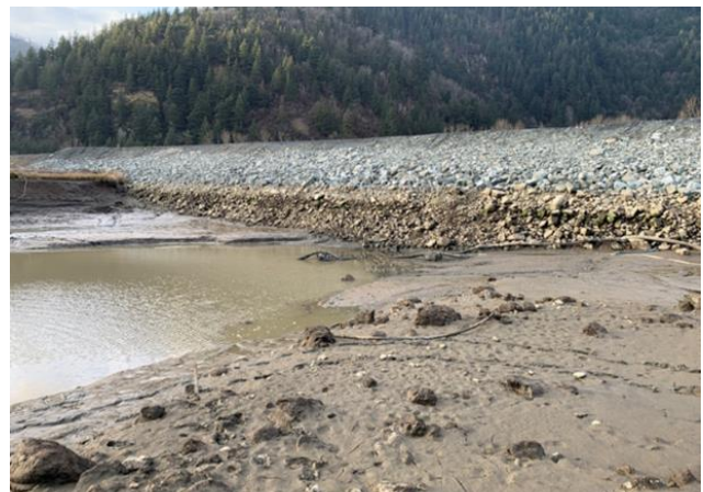
Fig 18. Drained scour hole and exposed water side slope of dike breach repair.
