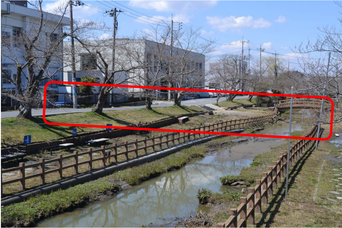
Utility & roadway damage along filled historic channel (GEER 2011)
